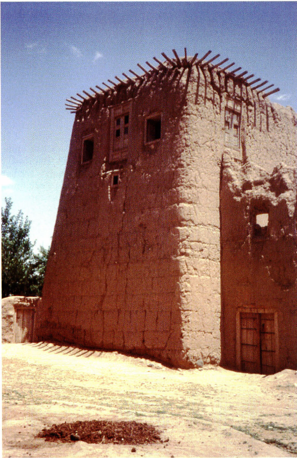
a: In Afghanistan, close to the border of Pakistan, an example of local typical fortified rural houses, or farms, built in “cob”. This building culture, in numerous regions of Afghanistan, is much more present than the adobe construction and locally called “ parsha ”.
