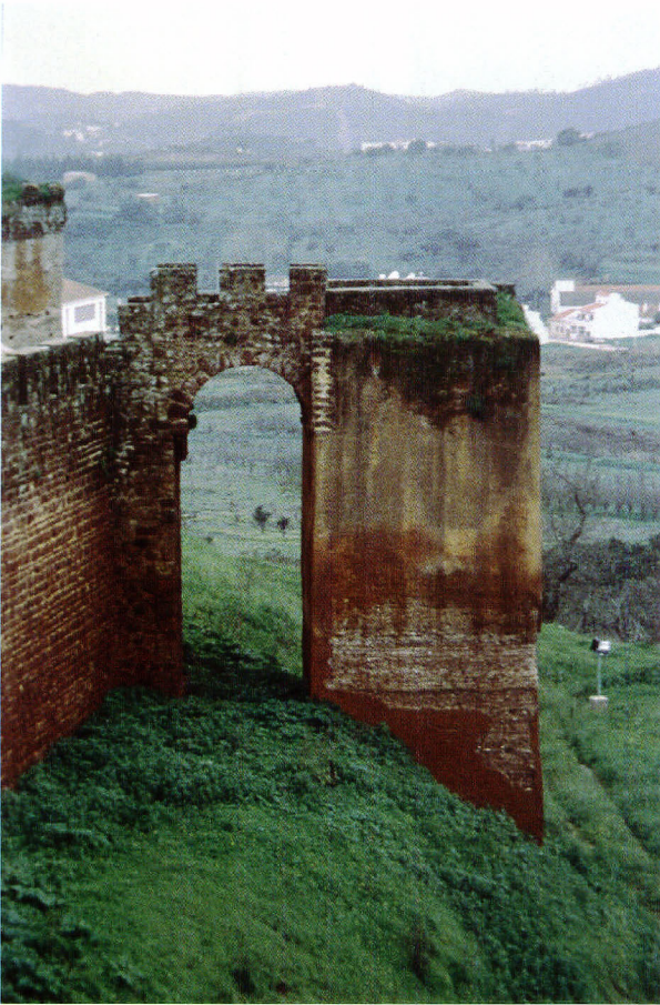
a: The remains of the Castle of Silves, Province of Algarve, South of Portugal. The tradition of fortified castles tracing back to the period of “ Al-Andalus ” (Moore times) testifying of the construction in “ pisé ” (“ taipa ”) is quite common in this region of Portugal where several projects of conservation have been launched.
