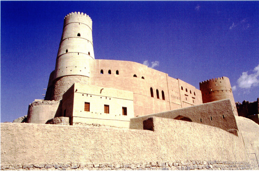
a: An aspect of a recent intervention of restoration which has been recently conducted on the Fort of Bahla, Sultanate of Oman, under the site guidance of Arch. Enrico d'Errico within the project carried out by the Ministry of National Heritage and Culture and the expertise of UNESCO. Here we can observe the partial restoration and reconstruction of the “ Borj ar-Rih ”, or “Wind tower”, according the architectural evidence given by a documentation coming from photographs taken at the end of the XIX th Century by a British explorer, Colonel Miles. All outer plasters have been made in traditional “ sarooj ” and earth and straw.
